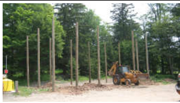
(Above) The initial construction phase of the Vehicle Storage Building has begun (July 2008)
